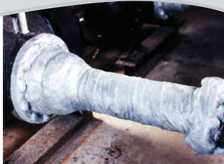
A sweating meter run pipe protected with Wax-Tape® #2A wrap demonstrates the wrap's ability to protect in wet conditions.
